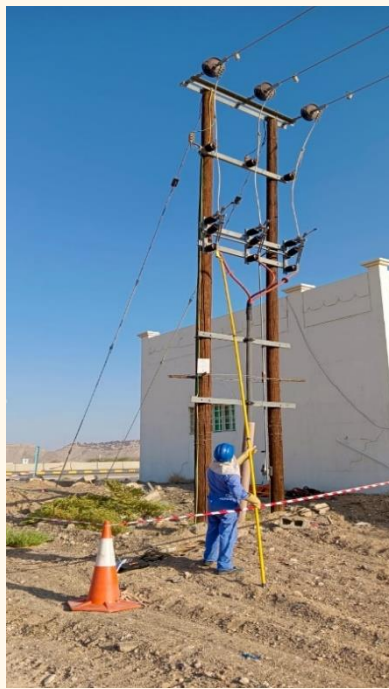
11KV & 0.415 KV Maintenance Services for Dhank, Yanqul, Al Sunayna, Al Mazam at Al Dhahirah Governorate for the period 2014-2017 (Completed)
