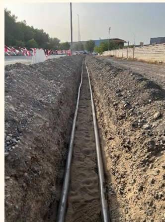
TENDER No: 04/2022,Construction of 11KV Interlink Feeder's to SIE-2 Primary Substation at North Batinah Governorate (Completed)
