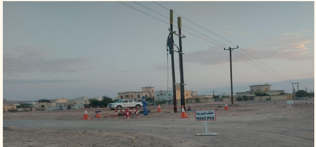
Tender No: NEDC-2023-062 & 084 Replacement Of Unsafe And Aged 11kv And 0.415kv Assets In Yanqul & Ibri Zone-2 At Al Dhahirah Governorate (Ongoing)
