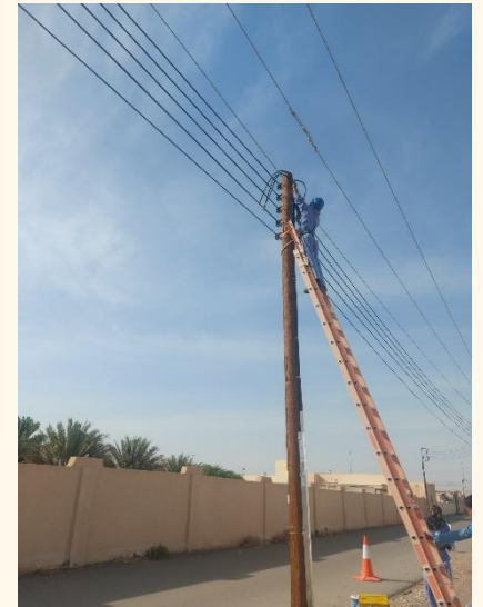
11KV & 0.415 KV Maintenance Services at Buraimi Governorate for the period 2018-2020(Completed)
