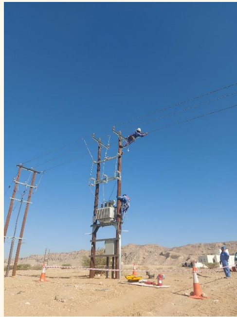
TENDER No: 02/2020 Re-Inforcement Work On Various Locations In Ibri Area Phase 2 At Al Dhahira Governorate(Completed)
