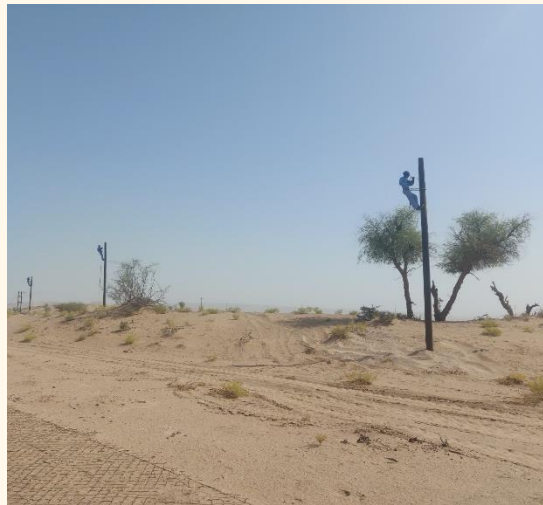
TENDER No: 84/2021, 126/2021 Extension of Power Supply to various agricultural plots at Al Dhahirah Governorate (Completed)
