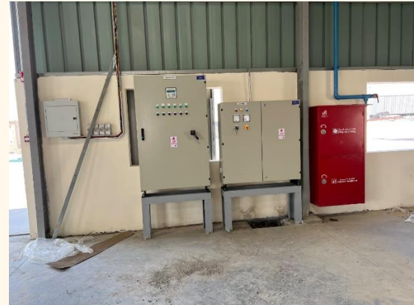
Installation SMDB Panels and cable Laying inside for Various Machinery at Stone World International and Zawaya stones in Sohar Industrial Area Phase 7(Completed)
